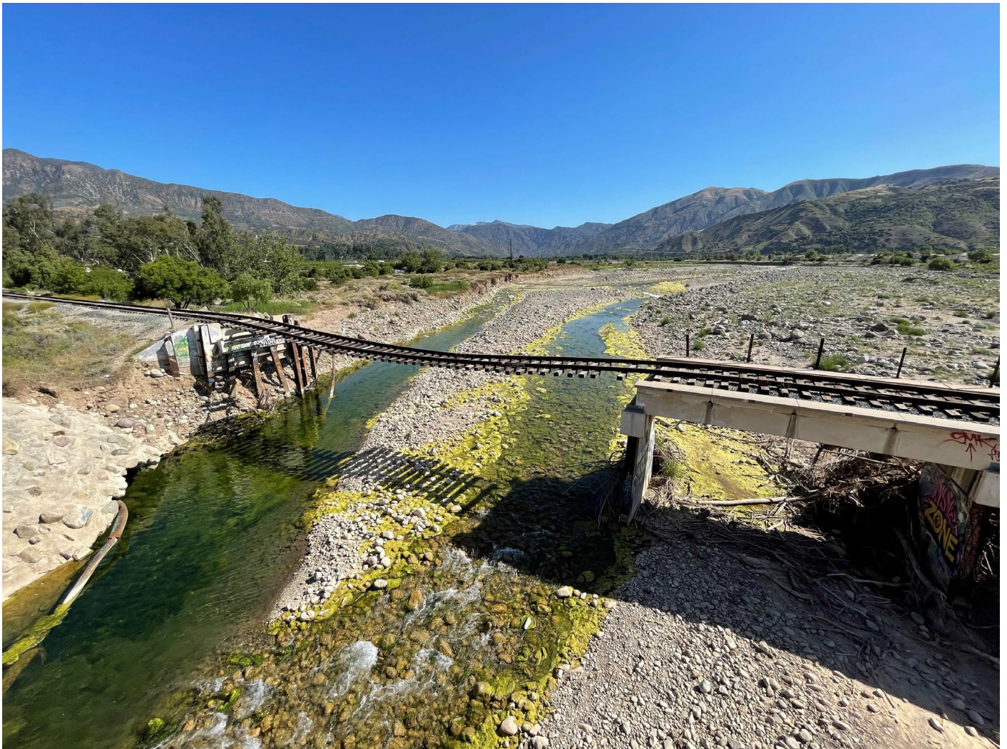
Figure 1 Damaged Portion of Railroad Bridge (looking upstream)
