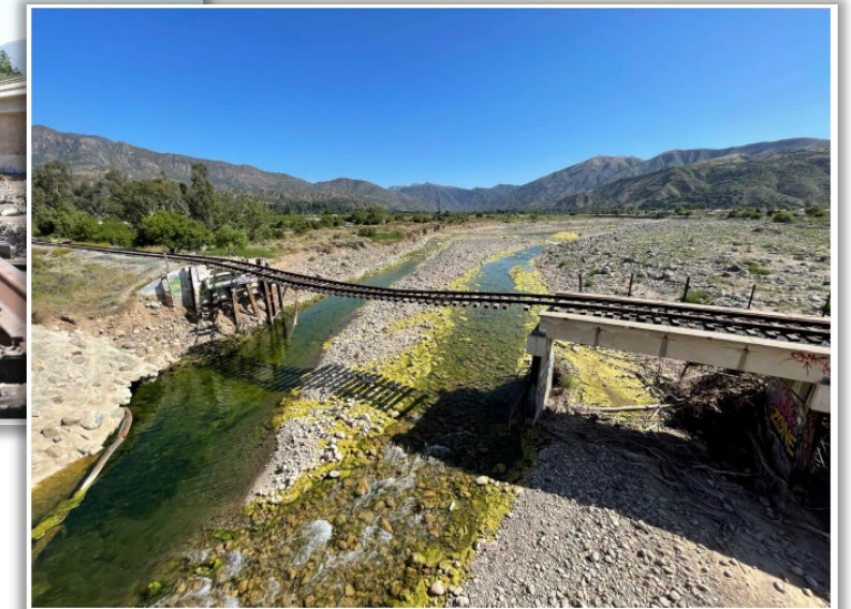
Figure 1 Damaged Portion of Railroad Bridge (looking upstream)
